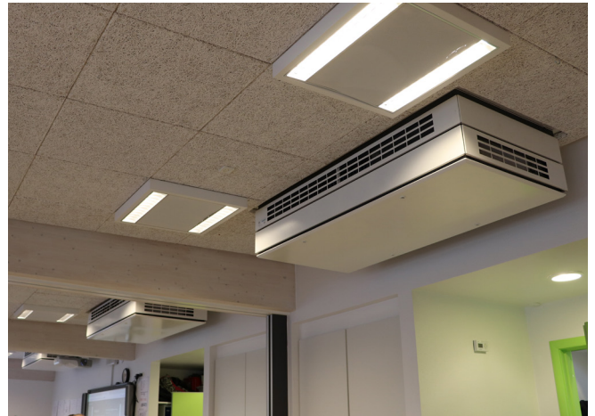
AM 500 ventilation units were installed throughout the school. The airflow from the four ventilation units is not obstructed by beams or lamps.
